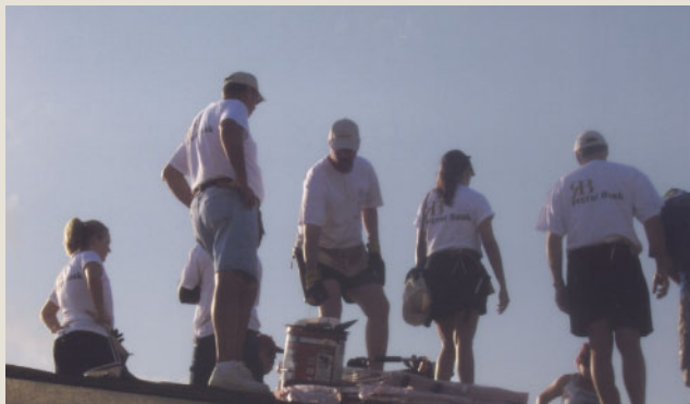
Bank employees put a roof on a Habitat for Humanity house in 2006.
